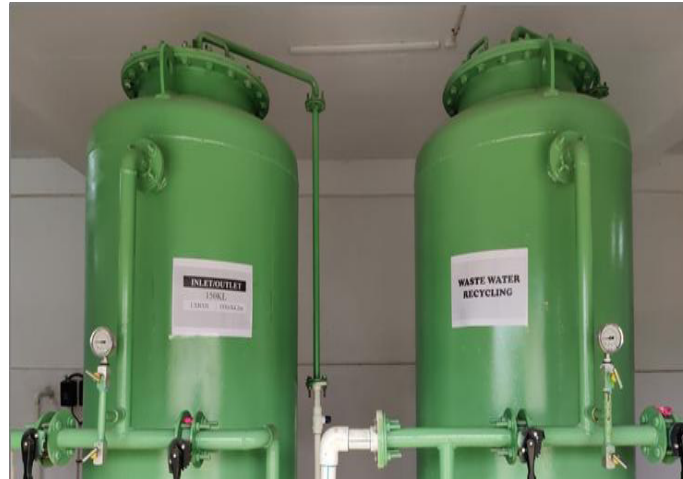
Figure 6. Sewage Treatment Plant
